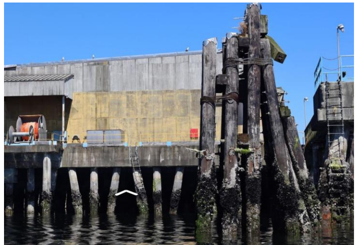
Figure 31 - Creosote pilings were often found as part of industrial overwater structures present in estuaries and the nearshore marine environment in the Cowichan Valley. Photo by Michael Miller Media (Resilient Coasts for Salmon imagery).
