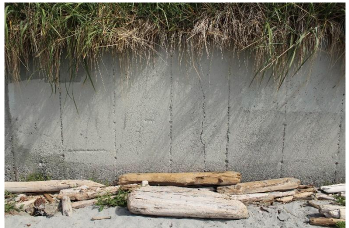
Figure 5 - An example of a seawall (one type of shoreline modification). Photo by Maria Catanzaro.
